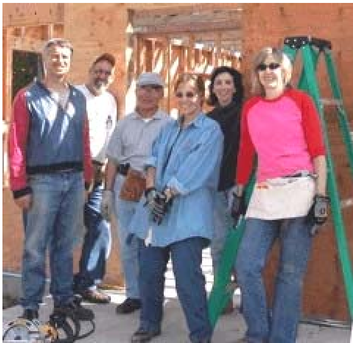
This group of volunteers, lead by Emil Kahut, left, and Construction Coordinator Dave Petrenka, second left, take a break from their hard work to smile for the camera. We rely on teams such as this group to get the job done.
