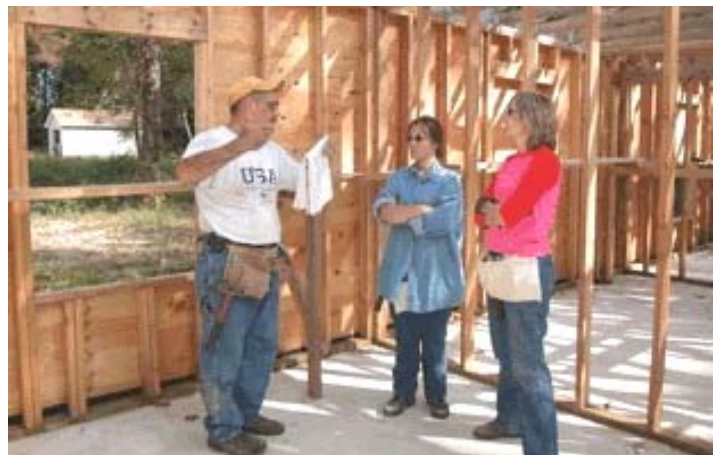
Construction Coordinator Dave Petrenka, left, explains the tasks of the day to volunteers on the work site on a Saturday this spring.
